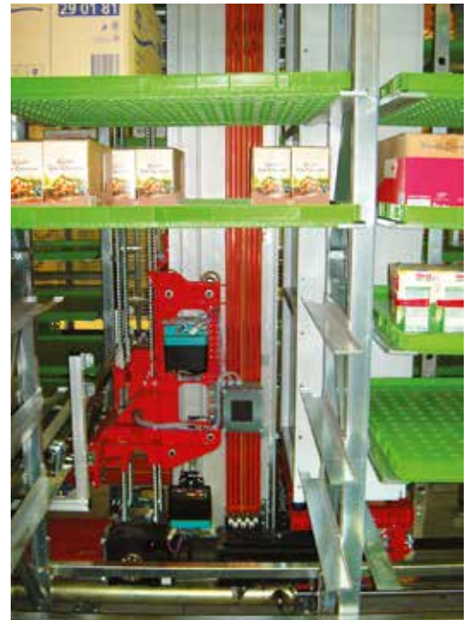
Mast conductor bar application (7-pole Pro-Ductor system) on mini-load
