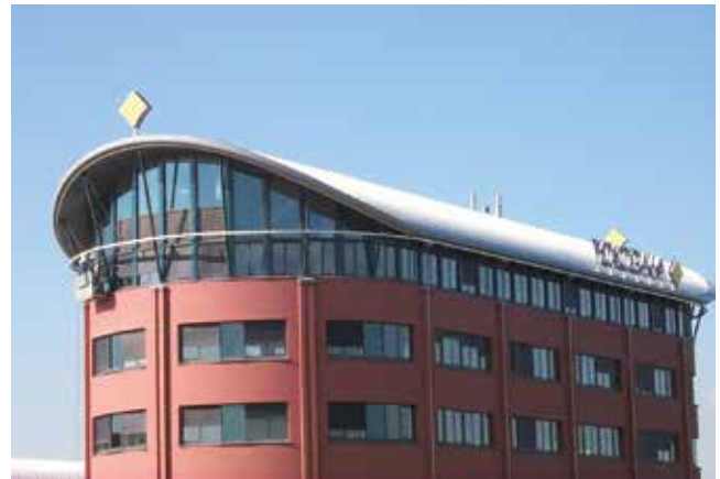
Curved installation for window cleaning equipment
