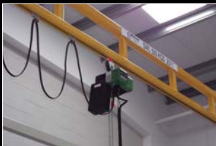
OVER HEAD CRANES
